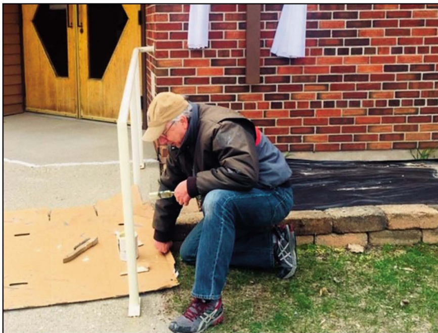
Father Stephen T. Rocker, pastor of St. Patrick's in Colton and St. Mary's in Potsdam, paints railings at St. Patrick's Church to pass time during the coronavirus isolation.
